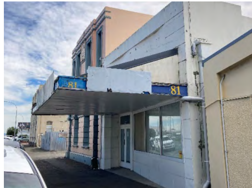
Deteriorating building. Childers Rd
