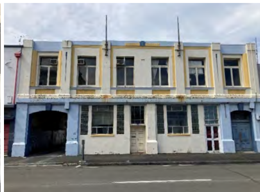
Deteriorating building. Lowe St
