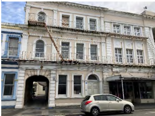
Masonic Hotel decaying façade. Lowe St
