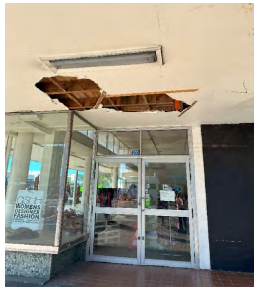
Main Street building decay. Gladstone Rd
