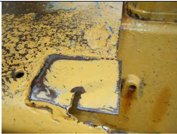
Sharp edges, protrusion, finger entrapment
