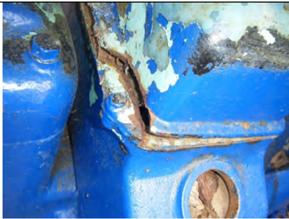
Sharp edges, rusted lifted parts
