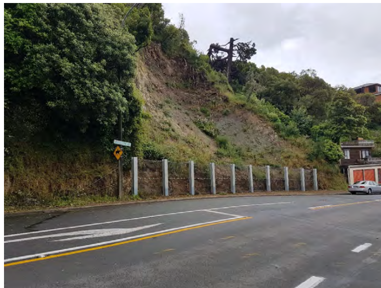
Figure 6-17: Example of rock fall protection fence installed at the toe of the slope
