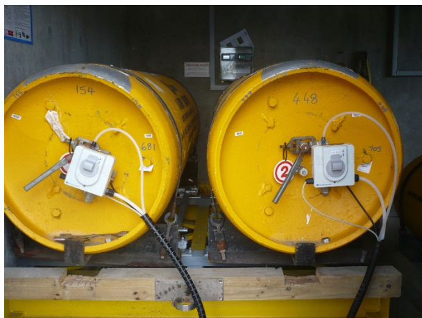
Figure 19. Gas chlorine drums
