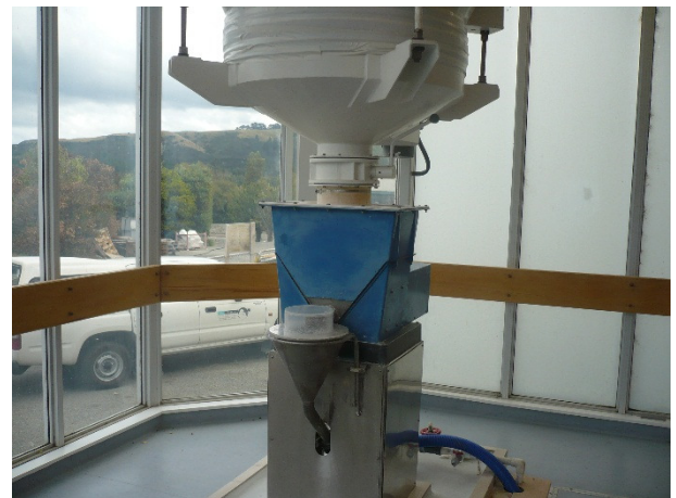
Figure 16. Lime feeder dosing point
