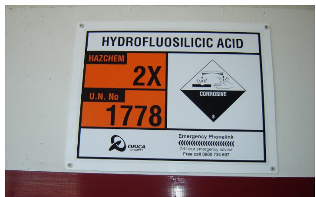
Figure 14. Fluoride dosing room
