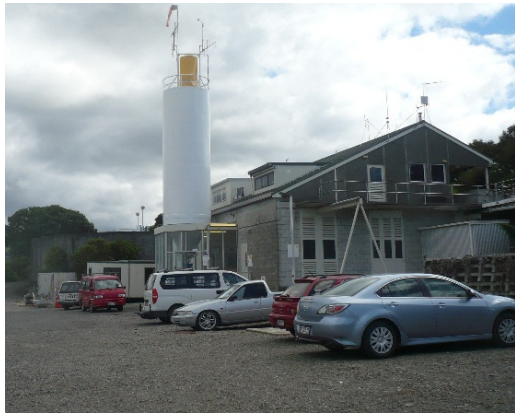
Figure 17. Plant building & lime storage tower
