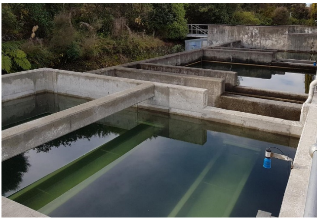
Figure 11. Rapid sand filters
