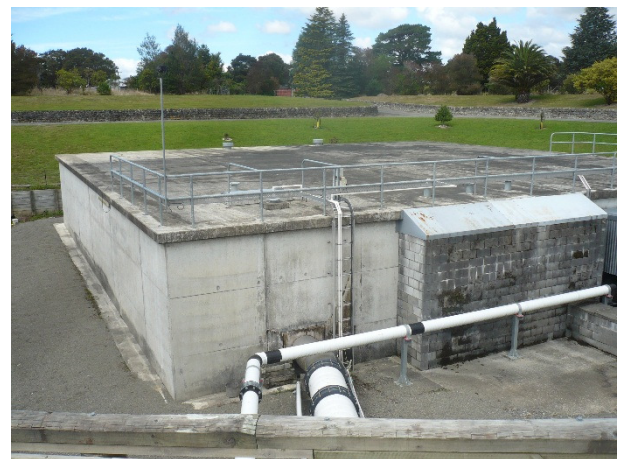
Figure 20. Treated water reservoir
