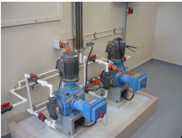
Figure 9. Coagulant (PACl) dosing
