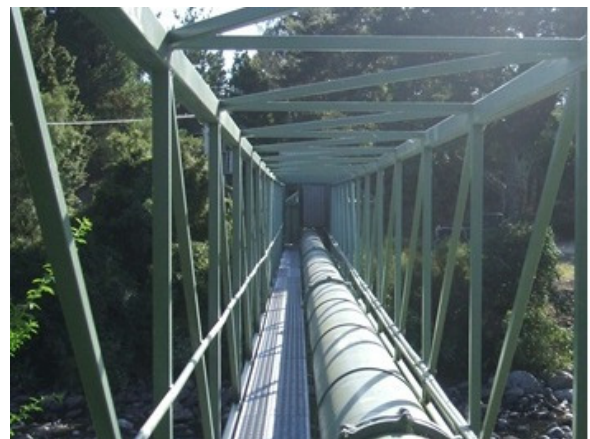
Figure 6. Raw water pipeline to WTP
