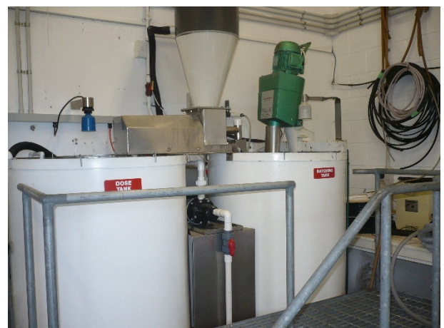
Figure 8. Polymer mixing facility
