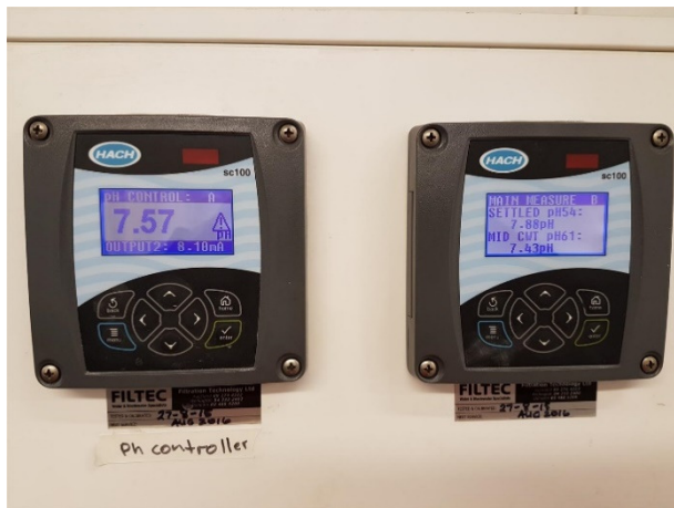
Figure 15. pH control to Lime feeder
