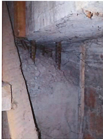
Figure 12c – Poor construction details evident in this beam to column joint
