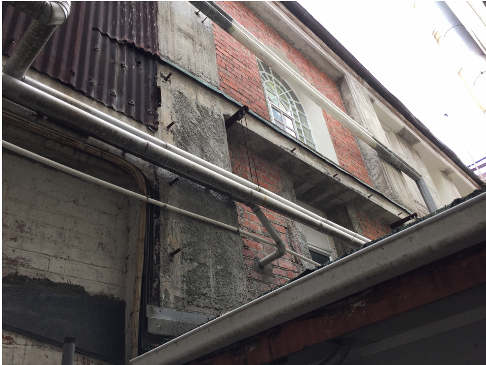
Figure 15 – External view of wall line at rear of Municipal building (shown in red in figure 13)
