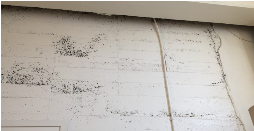
Figure 11 – View of hall extension "boney" concrete – poorly vibrated concrete resulting in exposed aggregate.
