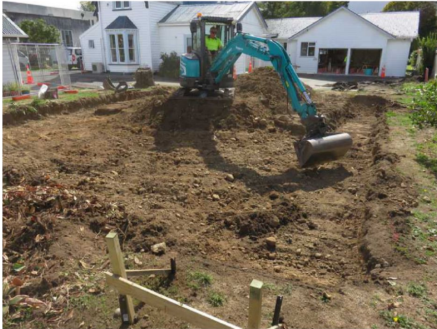
Illustration 1: Excavation for foundations for new residential units from Church Street facing north-east towards vicarage building (March 25th 2021).
